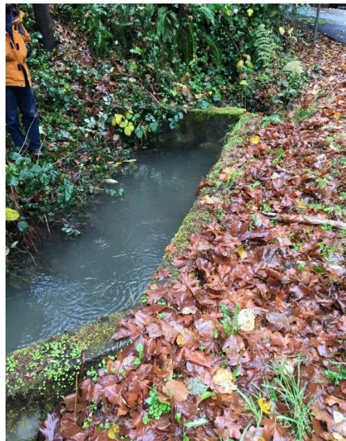
Beaver activity can result in system clogging and backwater conditions in stormwater infrastructure
