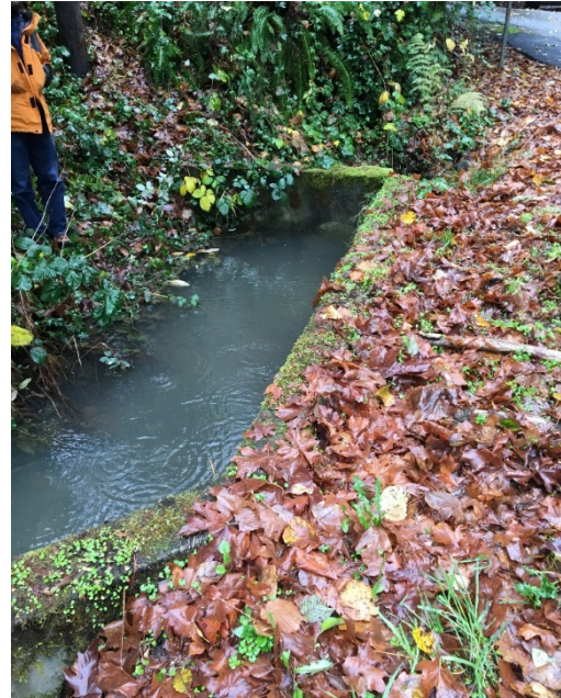
Beaver activity can result in system clogging and backwater conditions in stormwater infrastructure
