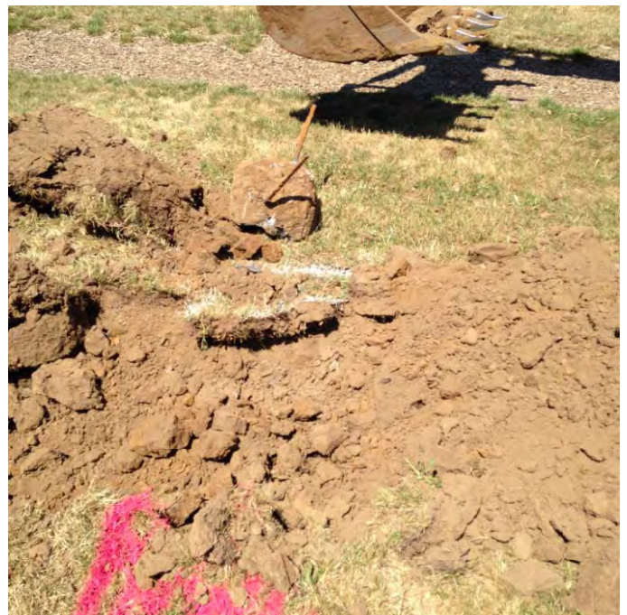
Photograph 4: Concrete debris encountered in test pit TP-9.
