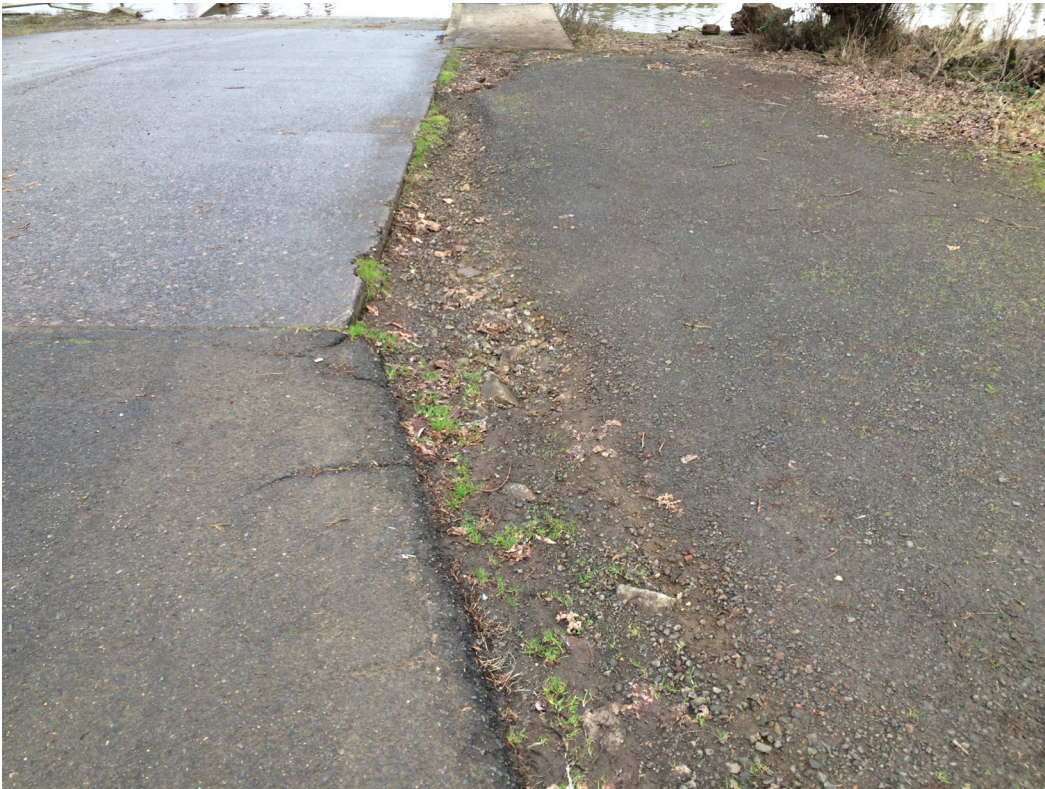
Photograph 10: Existing ramp and deteriorated walkway to ramp
