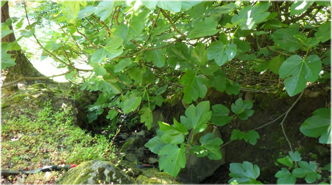
Photo Point 5. From the steep, eroded northeast drainage section facing northeast downstream
