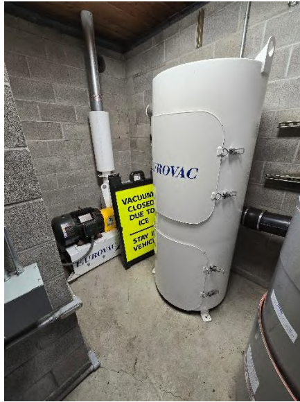
Vacuum Collector at Hillsboro
