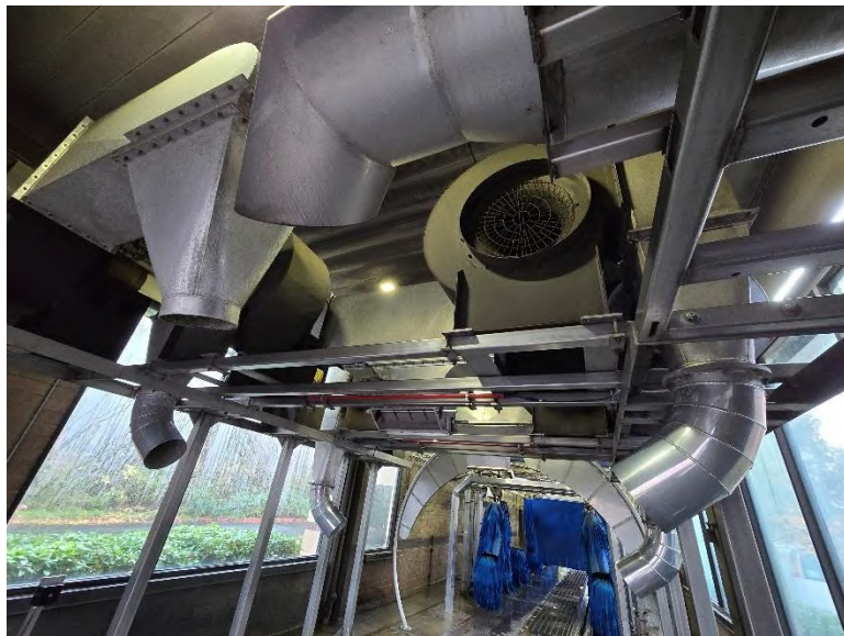
Blower equipment at Tualatin
