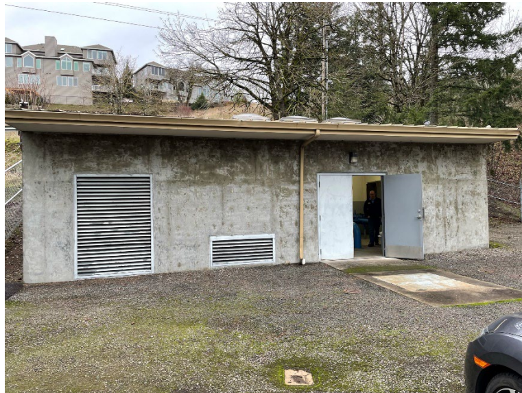
Photo 1-5 | Willamette Pump Station
