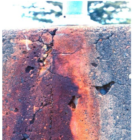
Figure 4-4. Guardrail Anchorage Corrosion
