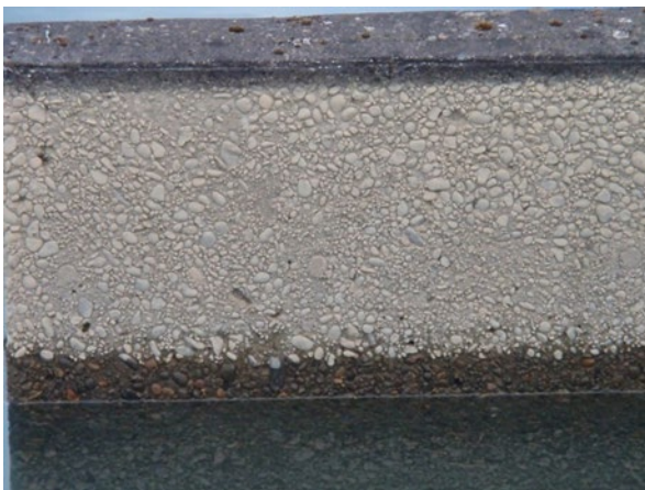
Figure 4-5. Flocculation/Sedimentation Basin Interior Wall
