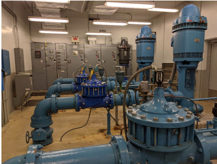
Photo 1-1 | Bolton Pump Station
