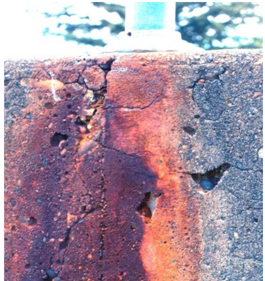
Figure 4-4. Guardrail Anchorage Corrosion
