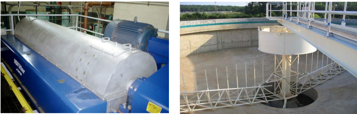
Figure 2-14. Example Photographs of a Centrifuge Dewatering Unit (left) and an Empty Gravity Thickener (right)
