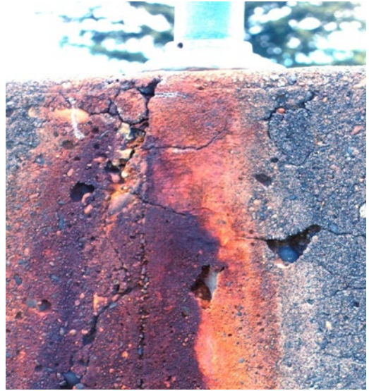
Figure 4-4. Guardrail Anchorage Corrosion
