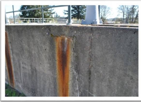
Figure 6-9. Sedimentation Basins Concrete
