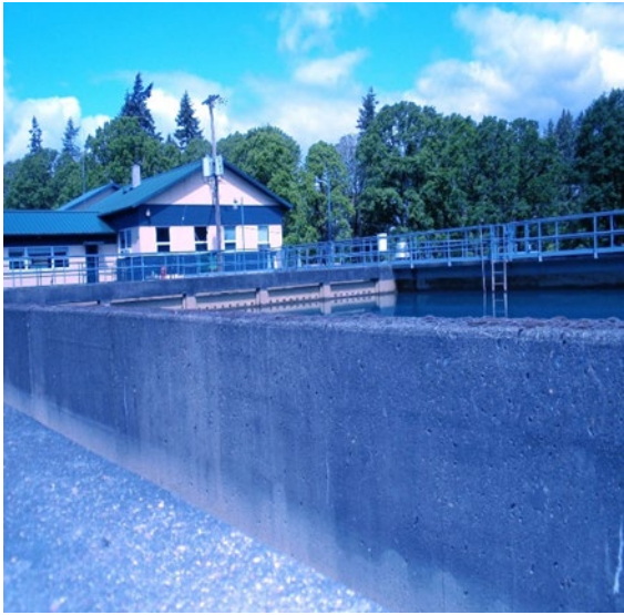
Figure 4-3. Flocculation/Sedimentation Basin South Wall
