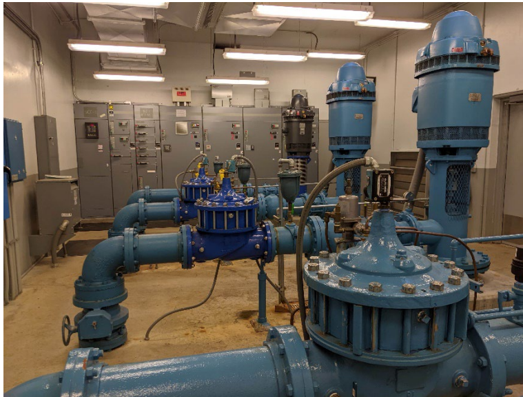
Photo 1-1 | Bolton Pump Station
