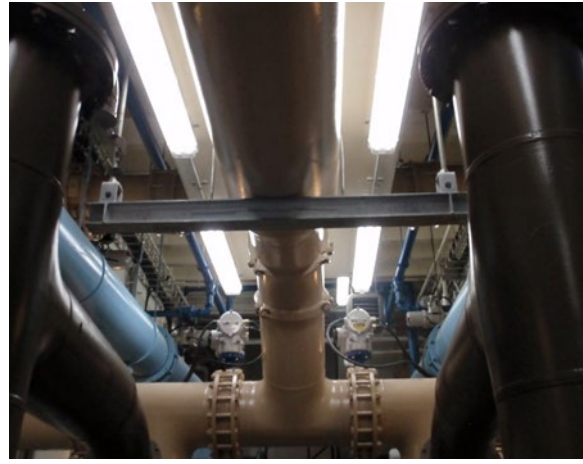
Figure 4-2. Filters Pipe Gallery
