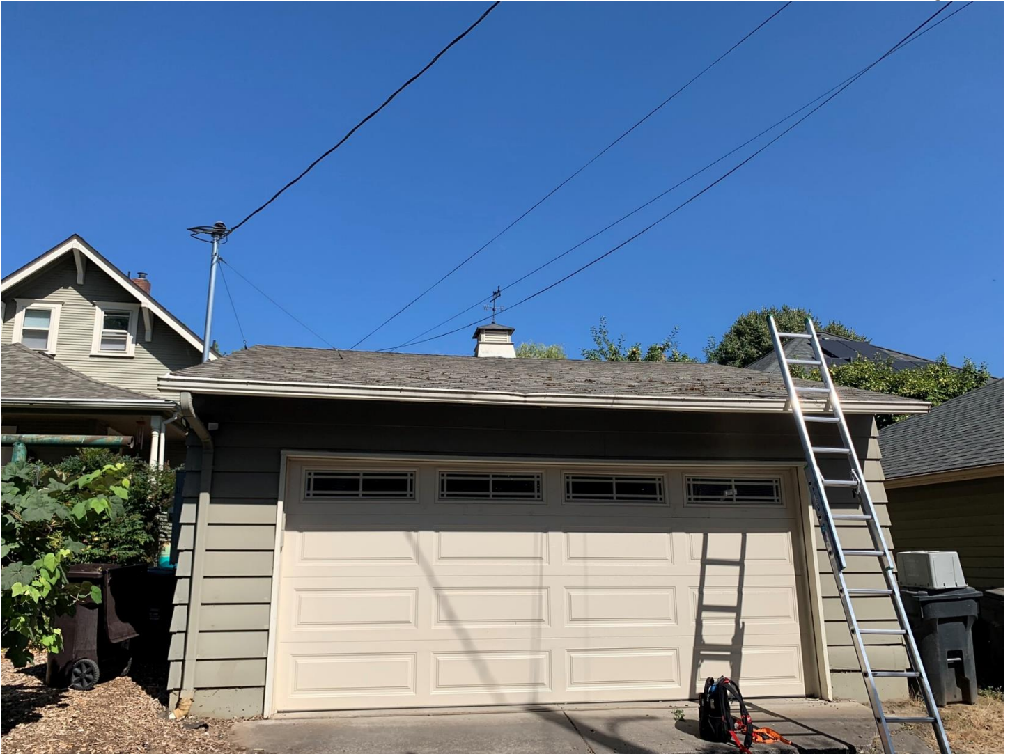
Figure 7: View of the rear of the garage from a position directly across the alley from the garage
