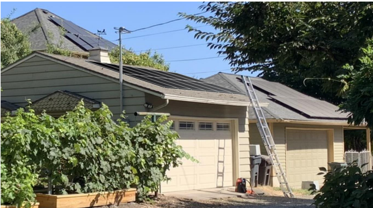
Figure 3: Garage roof as visible from the alley, with the 12 module array drawn on the roof. Note that the neighboring property has solar modules on the rear-facing roof plane.
