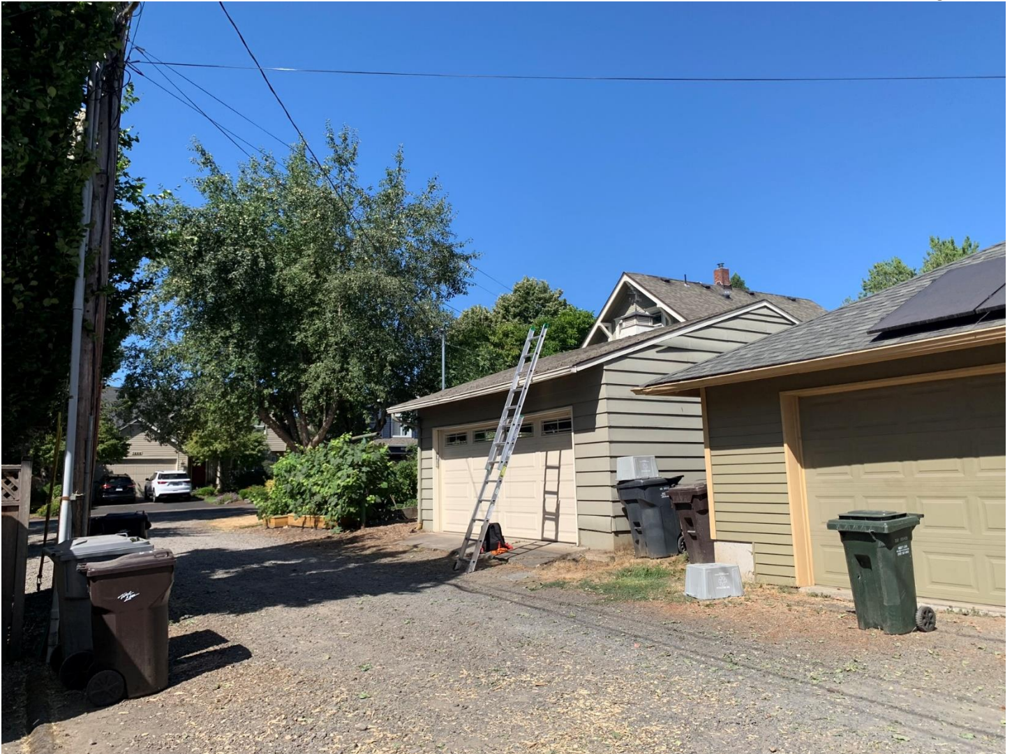
Figure 6: View of the rear roof of the garage from a garage on the opposite side of the alley
