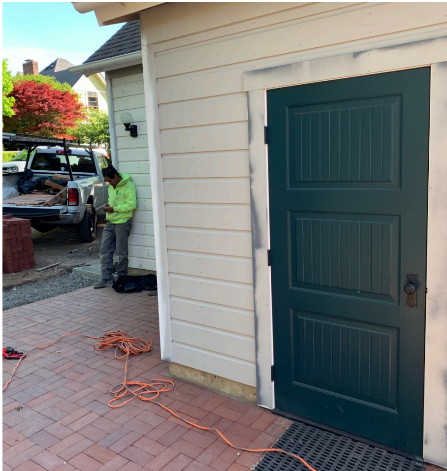
Side Facing façade – Door shown on right to be filled in with matching siding.
