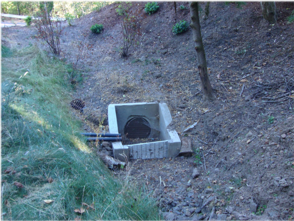
Photo Point 1. From the lower end of the drainage facing north toward the newly constructed storm drain.
