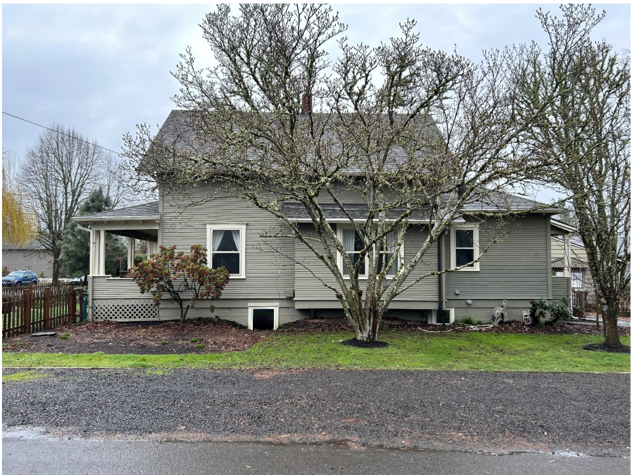
Side Facing façade (15 th Street) – window to be replaced at lower right.
