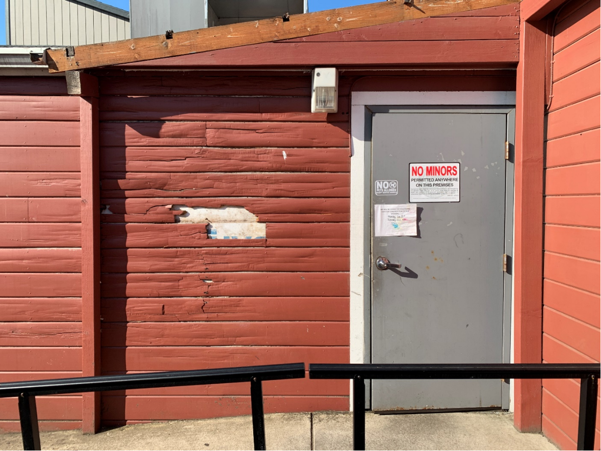
Damaged siding in rear courtyard.
