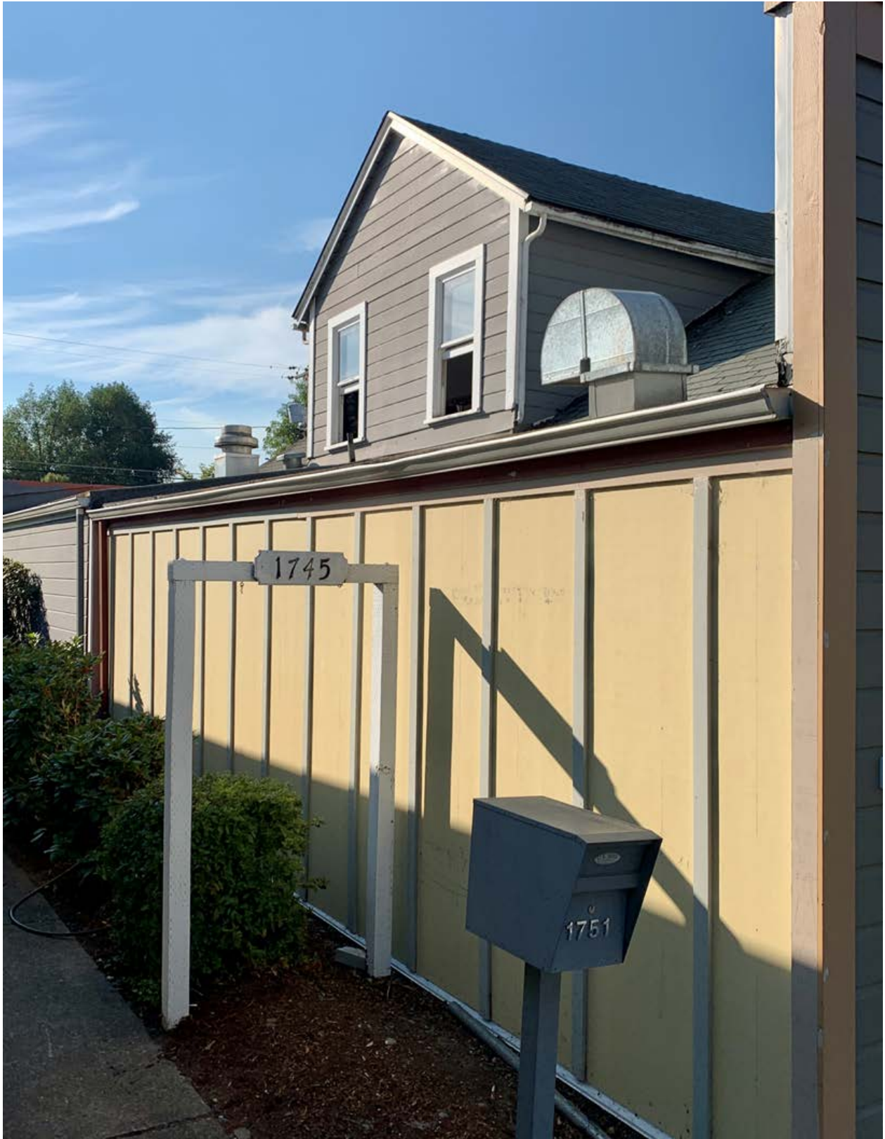
Existing side (east) façade as seen from sidewalk along Willamette Falls Drive.
