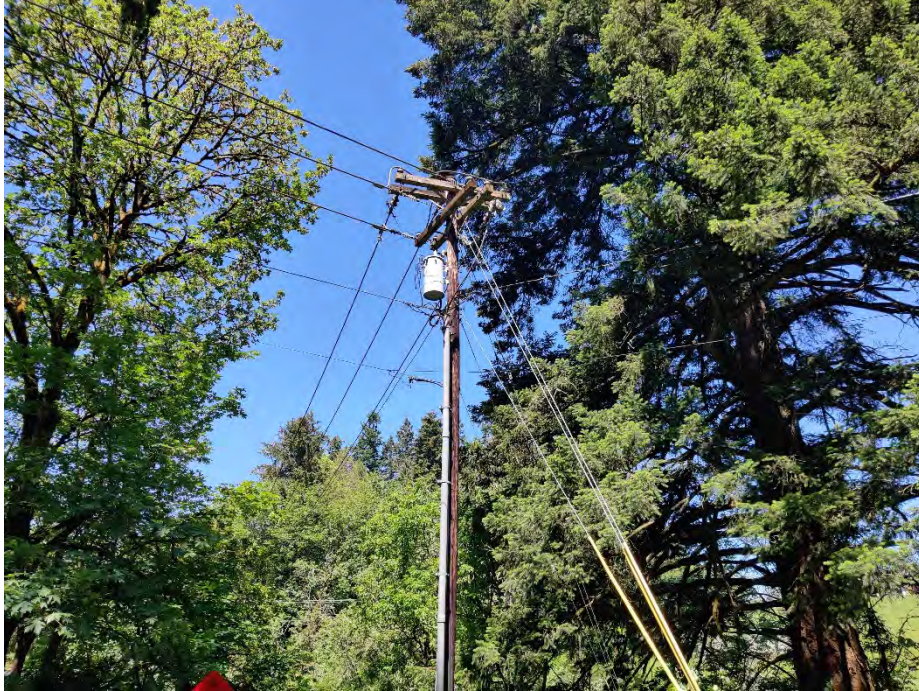
Photo 15. Pole mounted transformer in the northwest corner near the Tualatin River
