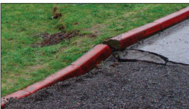
Street and ground cracks. Photo credit: Scott Burns.
