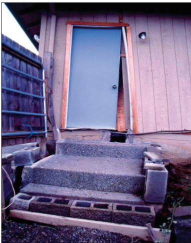
House cracks. Photo credit: Scott Burns.
