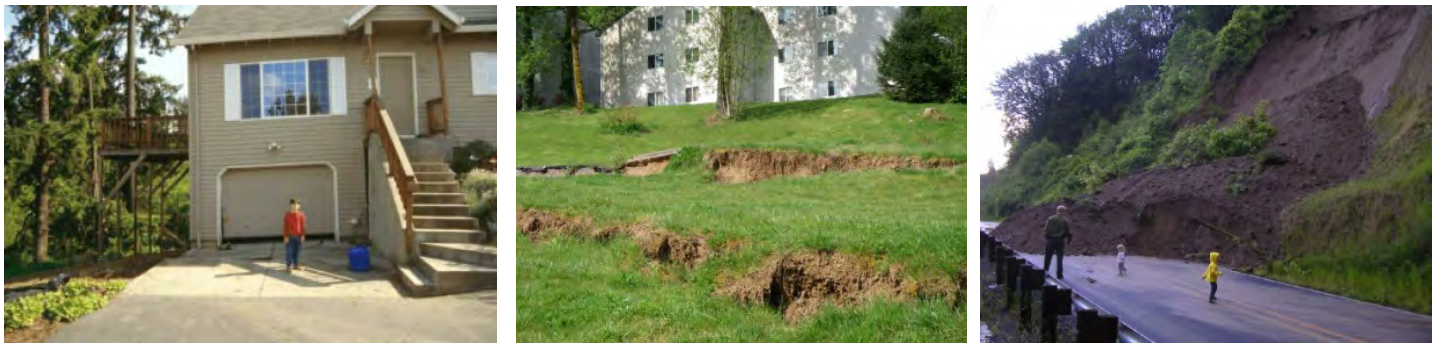
Figure 33. Photographs of historic landslide damage.
