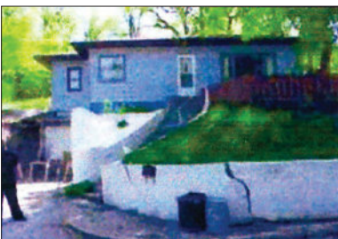
Foundation cracks. Photo credit: FEMA www.fema.gov .
