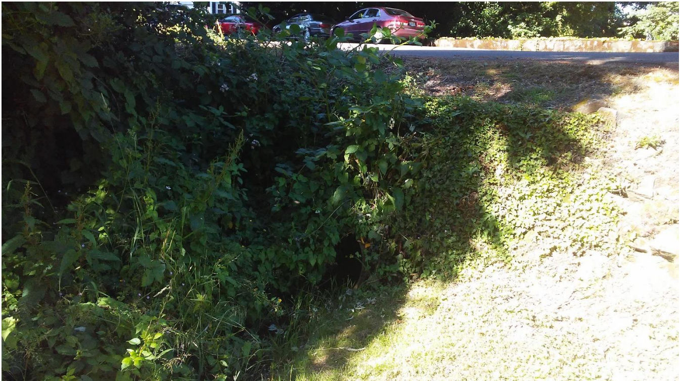
Figure 2. Cascade Pond Creek looking downstream at the River St. culvert inlet (30" diam).
