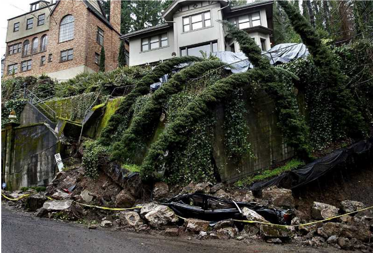
PAMPLIN MEDIA GROUP FILE PHOTO - Homeowners can begin to protect themselves from landslides by understanding how they work. This southwest Portland landslide occurred near a planned development.
