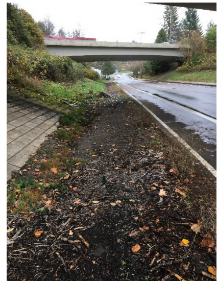
Flat topography and an insufficient stormwater collection system along Blankenship Road frequently results in ponded water and road closures during storms.
