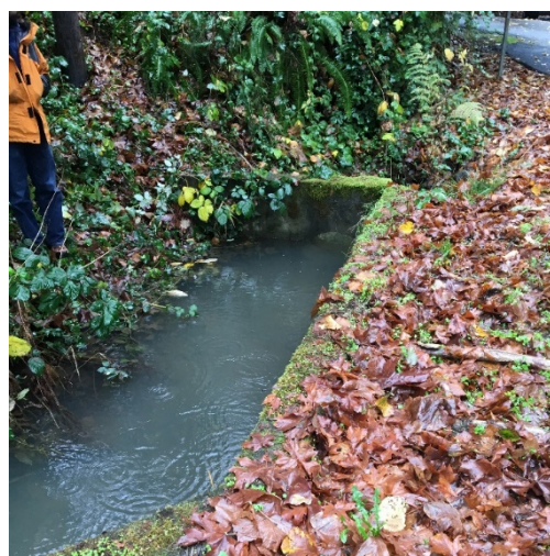
Beaver activity can result in system clogging and backwater conditions in stormwater infrastructure
