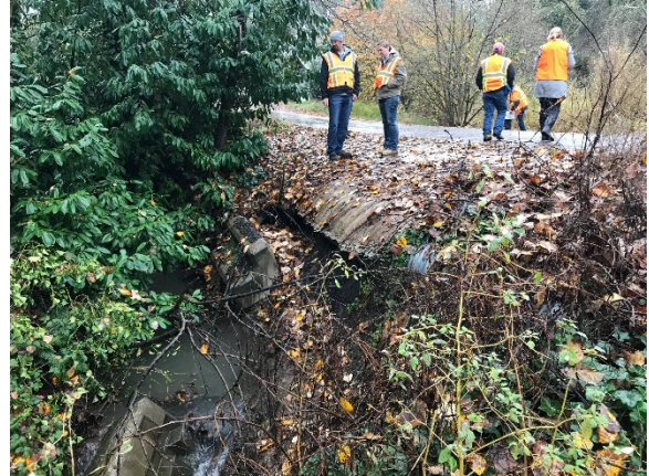
Identified system deficiencies include failing infrastructure as well as capacity limitations.
