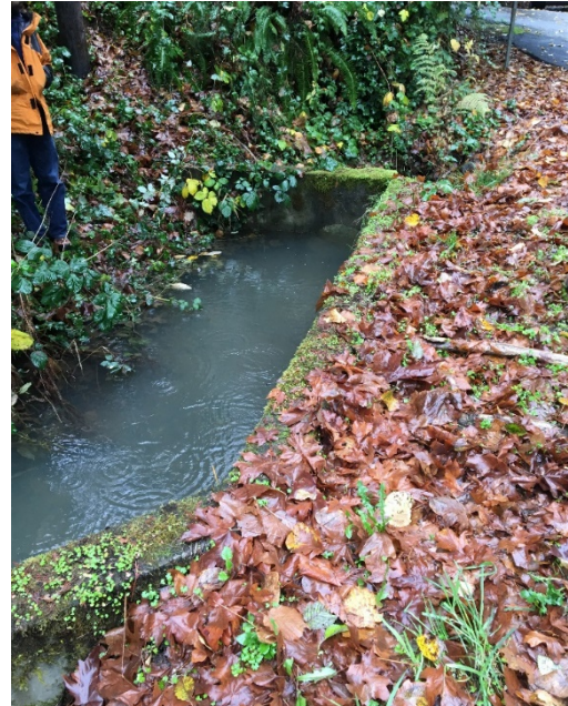
Beaver activity can result in system clogging and backwater conditions in stormwater infrastructure
