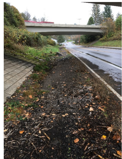
Flat topography and an insufficient stormwater collection system along Blankenship Road frequently results in ponded water and road closures during storms.
