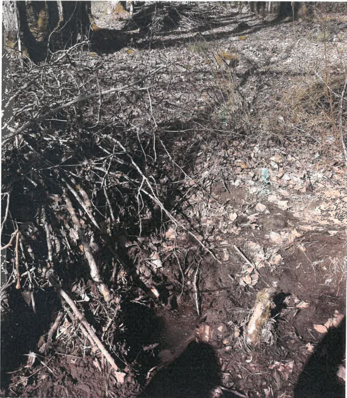
Photo 2. Water seeping from soil in the existing channel into a shallow excavation (bottom center of photo) near the junction of Tannler Drive and Blankenship Road on March 9, 2019. Photo taken looking upstream from near the road junction along the channel axis. The seepage indicates that the channel continues to transmit subsurface water despite the disconnection of the channel from upstream runoff.
