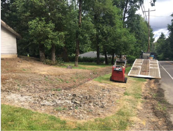
Photograph 1: Photograph taken in the central northeastern section of the site. Shows the locations of IT-1 and IT-2.
