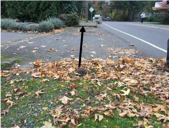
FIG-2 Existing circular area drain in Old River Road. Approximately 62 LF from catch basin. 12 inch concrete pipe found 1.9 feet below rim. Note that GIS maps note a drain where the mail boxes are. No drain was found. Road slopes vary between 2-5% per survey data.
