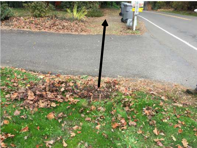
FIG-3 Existing rectangular area drain found approximately 121 LF from circular area drain. Note that rim is approximately 6 inches below adjacent pavement grade. 12 inch concrete pipe found 16 inches below rim grade. Pipe continues North. GIS Map shows an additional area drain/catch basin, but was not found during the site visit.
