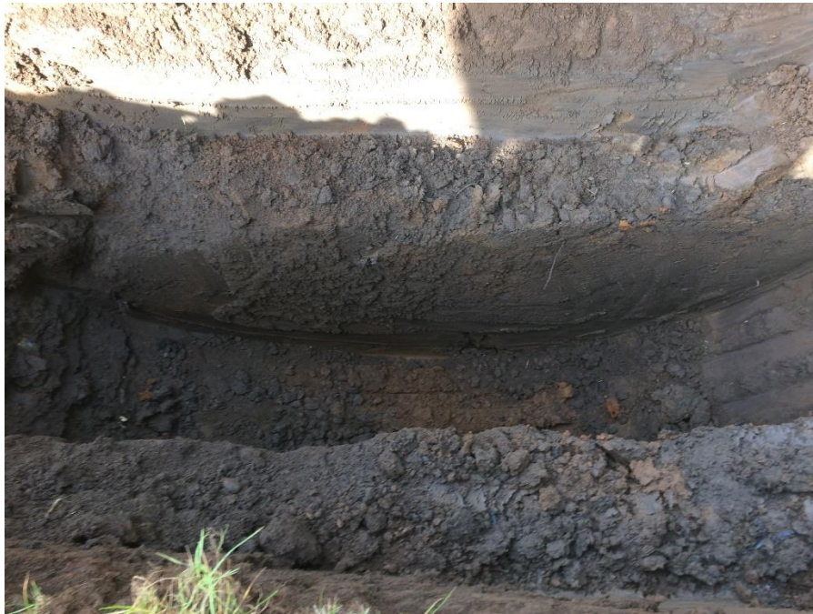
Undocumented Fill and Exposed Native Soils in Test Pit TP-2
