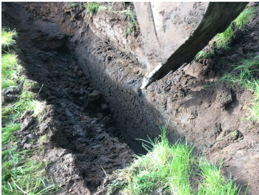
Undocumented Fill in Test Pit TP-2
