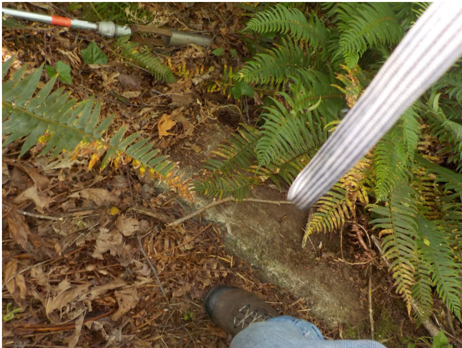
Photo 10 – Close-up view of weathered and partially buried concrete blocks observed near the southern portion of the site.
