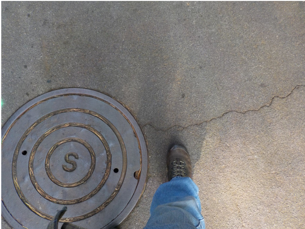
Photo 12 – View of cracking in surface of Wildwood Drive near site.
