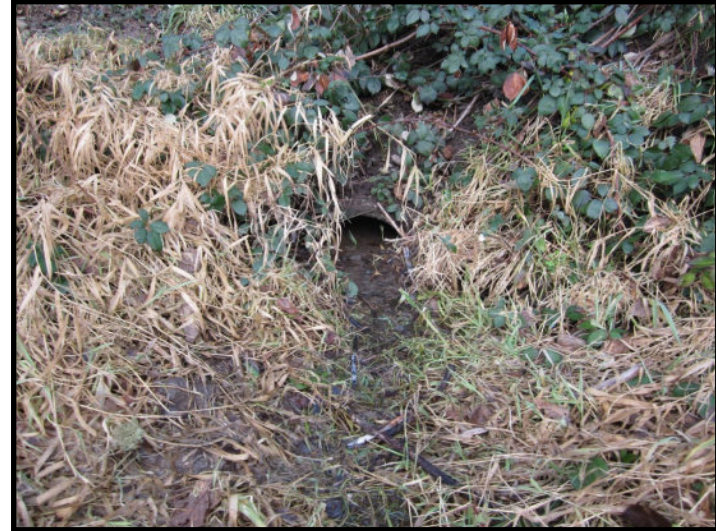
Photo B. View west of buried 12 inch concrete pipe draining stormwater from north into wetland.
