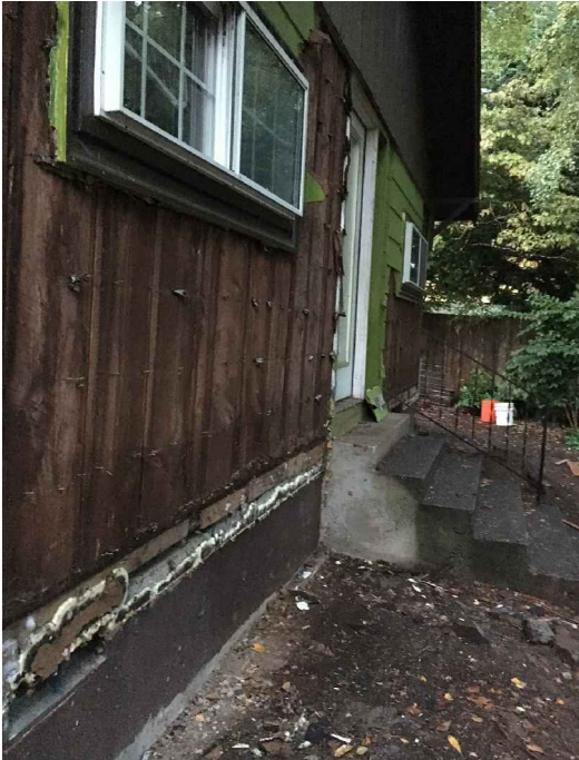
SOUTH WALL At Exterior Face of Sill Connection; Bottom or Boards Were Partly Exposed with Many Rotting and Deformed
