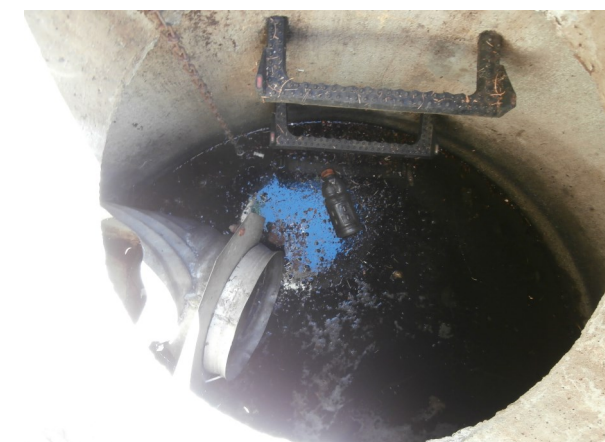
Existing Pollution Control Manhole trapping debris
