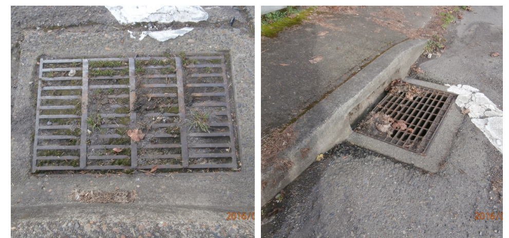
Many storm drains existing along OR 43 are in poor condition or clogged with debris
