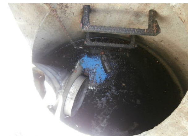
Existing Pollution Control Manhole trapping debris
