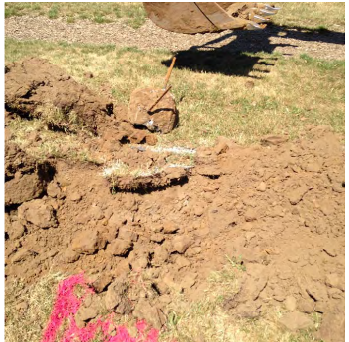
Photograph 4: Concrete debris encountered in test pit TP-9.
