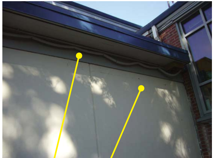
P1010392.JPG Electrical run on exterior. Cracks in concrete. (Building 'C')
