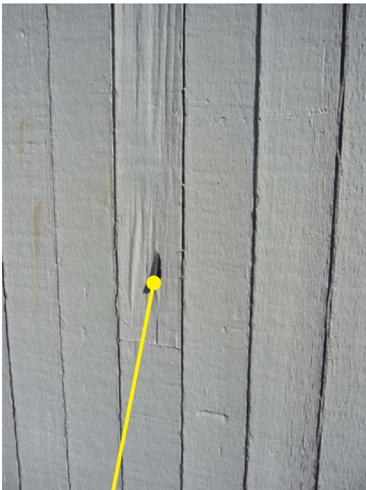
P1010382.JPG Peeling paint and dryrot on wood siding. (Building 'E')
