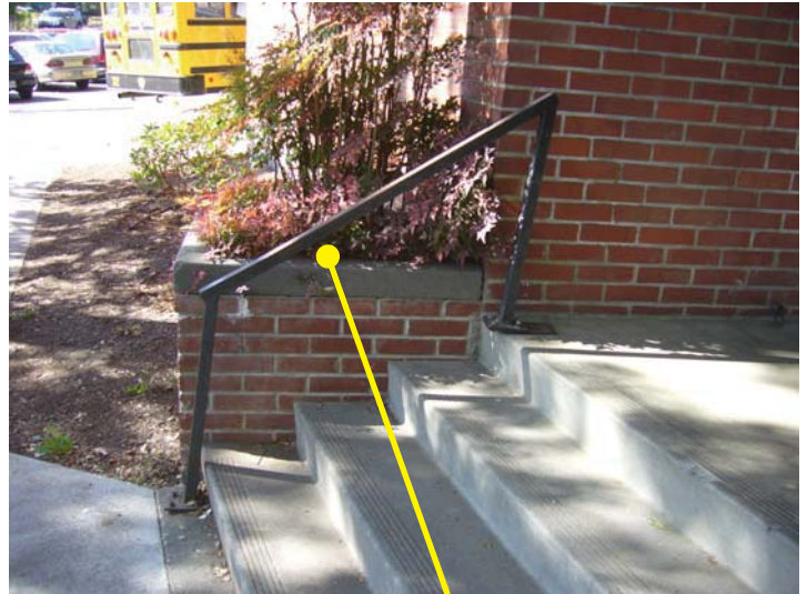
P1010390.JPG Substandard handrails. (Building 'B')
