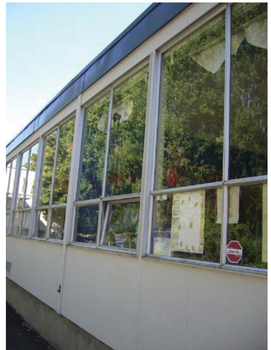
P1010383.JPG Old and energy inefficient aluminum windows. (Building 'E')
