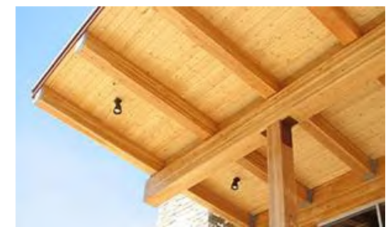
GLUE-LAMINATED WOOD BEAMS
