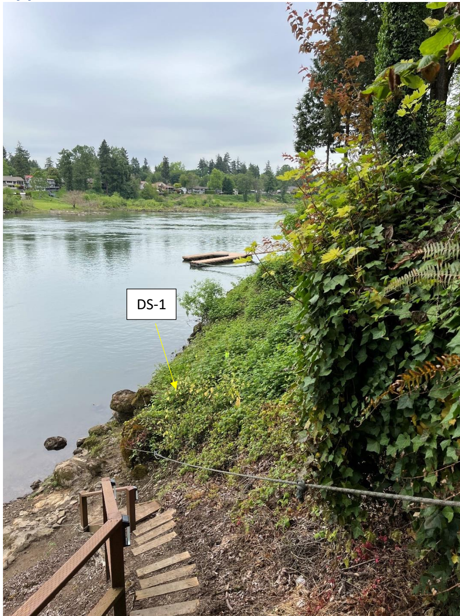
Figure 7a. Ground level photograph of cliff on Site between the house and Willamette River facing northeast; DS-1 is located within the toe slope between the cliff and the Willamette River. Flag presence is hard to spot due to vegetation growth. Note the boulders present.
