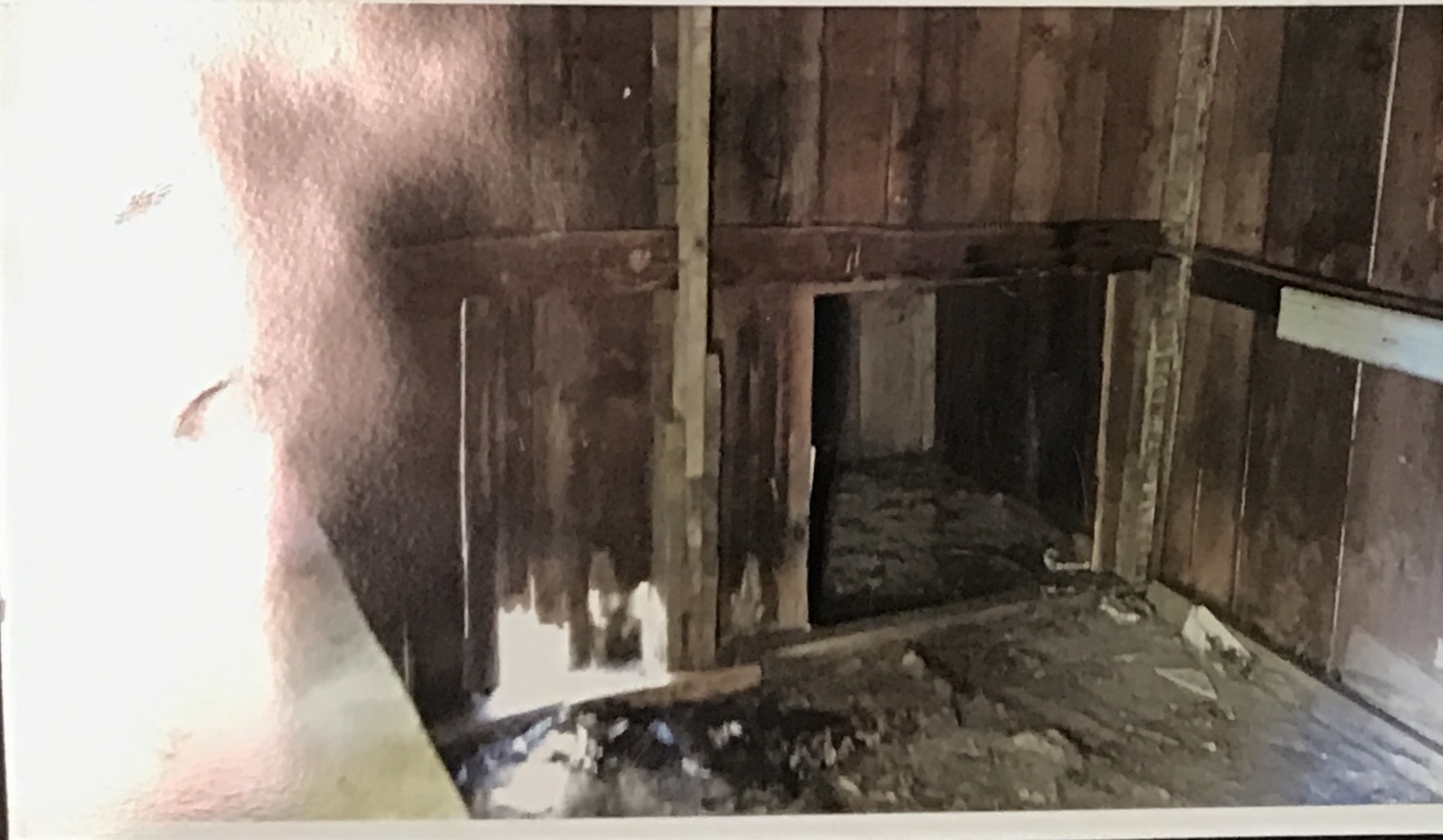
DIRT FLOOR / BUILT NO FOUNDATION / DIRECTLY ON SOIL
