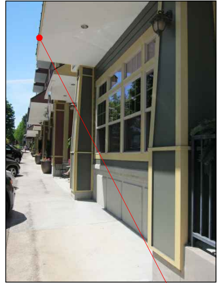
1980 WILLAMETTE FALLS DRIVE AWNING 24"+ FROM CURB
