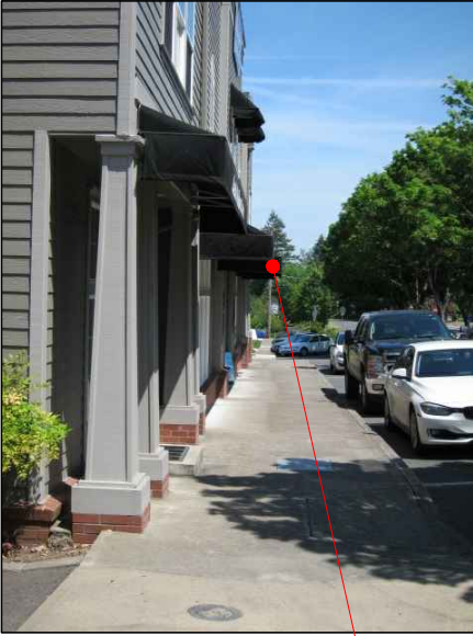
2008 WILLAMETTE FALLS DRIVE AWNING 48"+ FROM CURB
