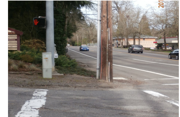
Marylhurst Drive at OR 43 traffic signal has no ADA accessibility at crossing and no sidewalks
