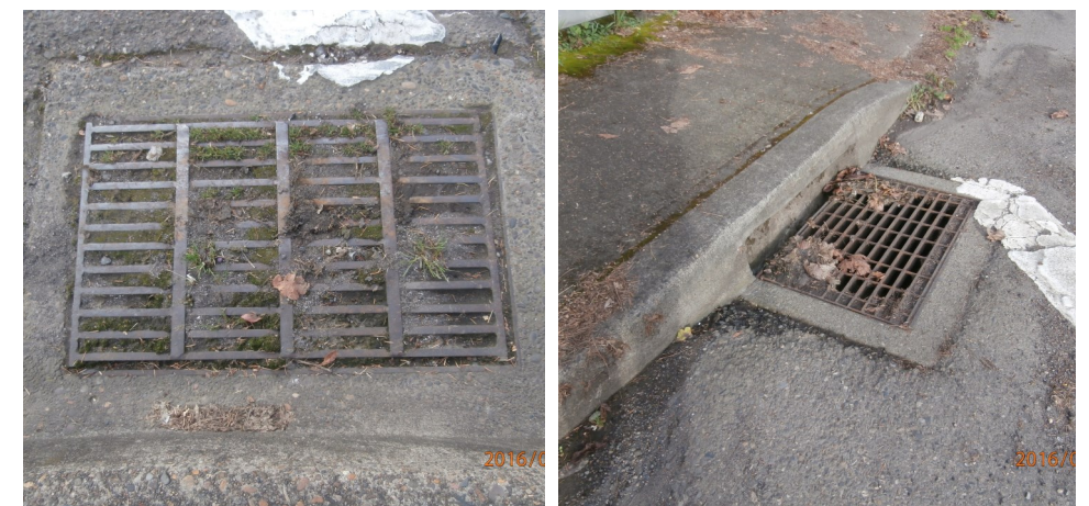
Many storm drains existing along OR 43 are in poor condition or clogged with debris
