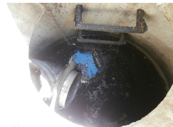
Existing Pollution Control Manhole trapping debris
